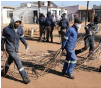
A JOINT City of Tshwane, SAPS and metro police operation to remove illegal electricity connections in Nellmapius. | JACQUES NAUDE African News Agency (ANA)
